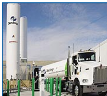
Distributed small scale natural gas liquefaction
