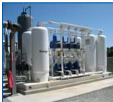
Biogas upgrading plants
